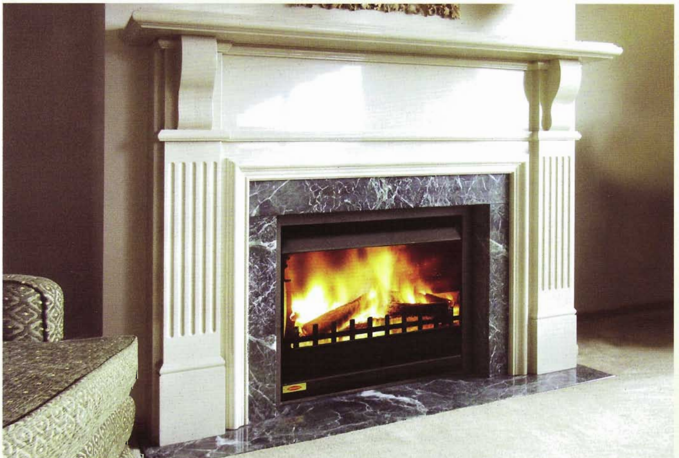
3. INSTALLATION COMPLETE: Jetmaster Universal, with marble margins, returns and hearth, and Pearce Dale 2-pack mantel
